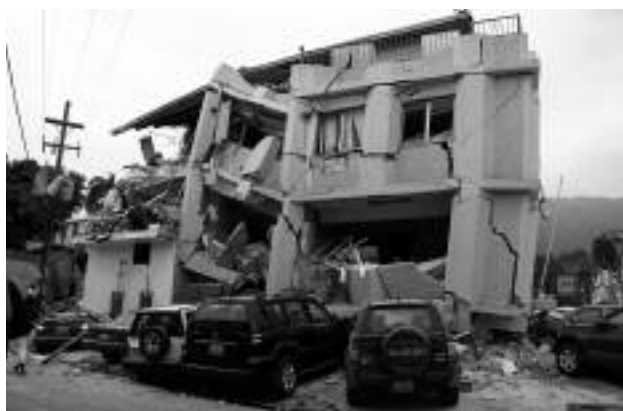
A quake-destroyed building in the streets of Port-au-Prince, Haiti on January 12, 2010.
